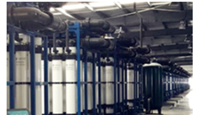
● Industrial wastewater treatment ●
