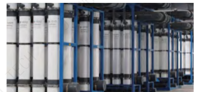
Zero Wastewater Discharge Project of a Paper Mill in Jiangsu
