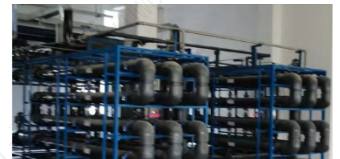
Zero Discharge and Hardness Removal Project of RO Concentrated Water in Guizhou
