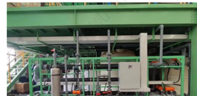
A Pharmaceutical Industry Material Removal Suspended Solids Project in Hunan
