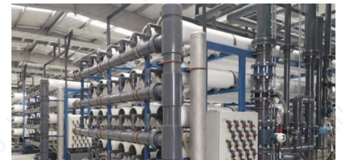
A Waste Salt Resource Utilization Project in Jiangsu
