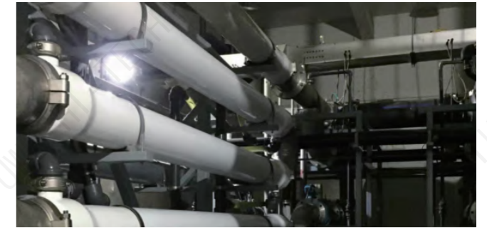
A Landfill Leachate Project in Chongqing
