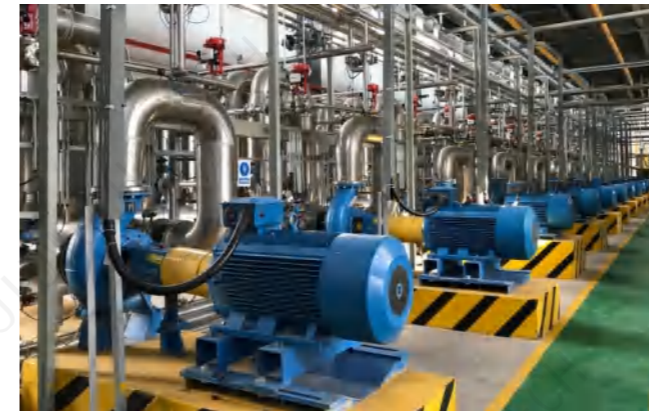
Ceramic membrane continuous filtration system of a threonine production enterprise in Inner Mongolia
