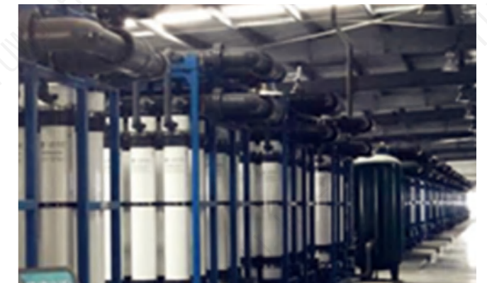
● Industrial wastewater treatment ●
